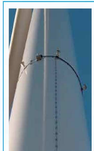
DTBird' Collision Avoidance Module Speakers installed on the WTG tower. 4 to 10 Speakers can be installed per WTG.
