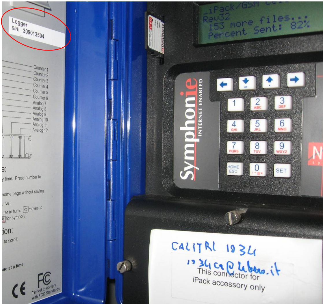
CALITRI met mast id# 1034. Photo showing: installed Logger NRG S/N: 309013504. The internet connection were working properly and wind data files were sent.
