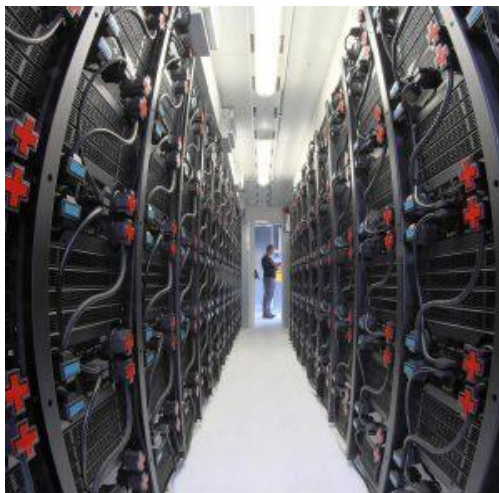
Fig. 3.35– Storage (BESS) interno del container
