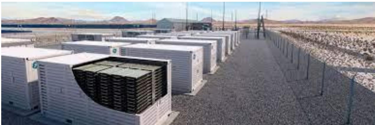
Fig.3.34 – Storage (BESS) in container in aree dedicate
