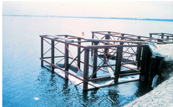
Figure 7. Example of unlevel weir boards and uneven effluent withdrawal across boards
