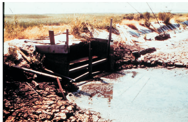
Figure 5. Nonfunctional weir boards
