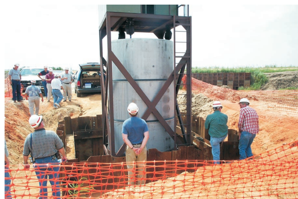
Figure 11. Extended telescoping cylinders at Blakeley
