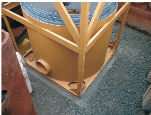
Figure 10. Anchor and foundation of telescoping weir
