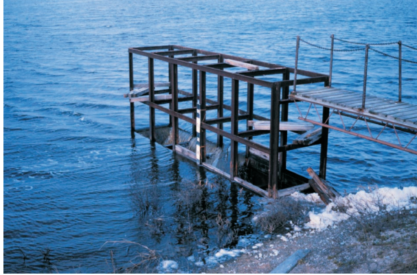
Figure 6. Example of potential safety hazard due to location of weir and boards
