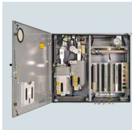
Control cabinet with the stored-energy spring mechanism
