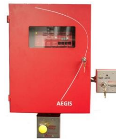
Fire suppression control panel
