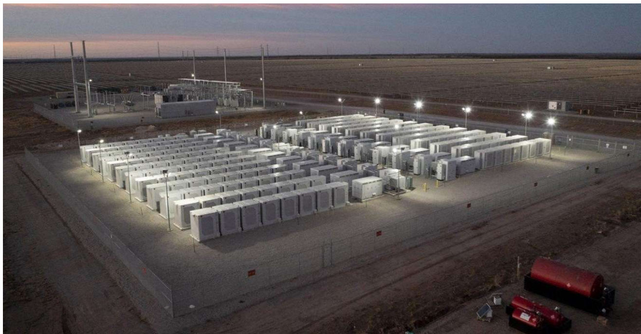
Fig. 3 – Stand-alone battery storage
