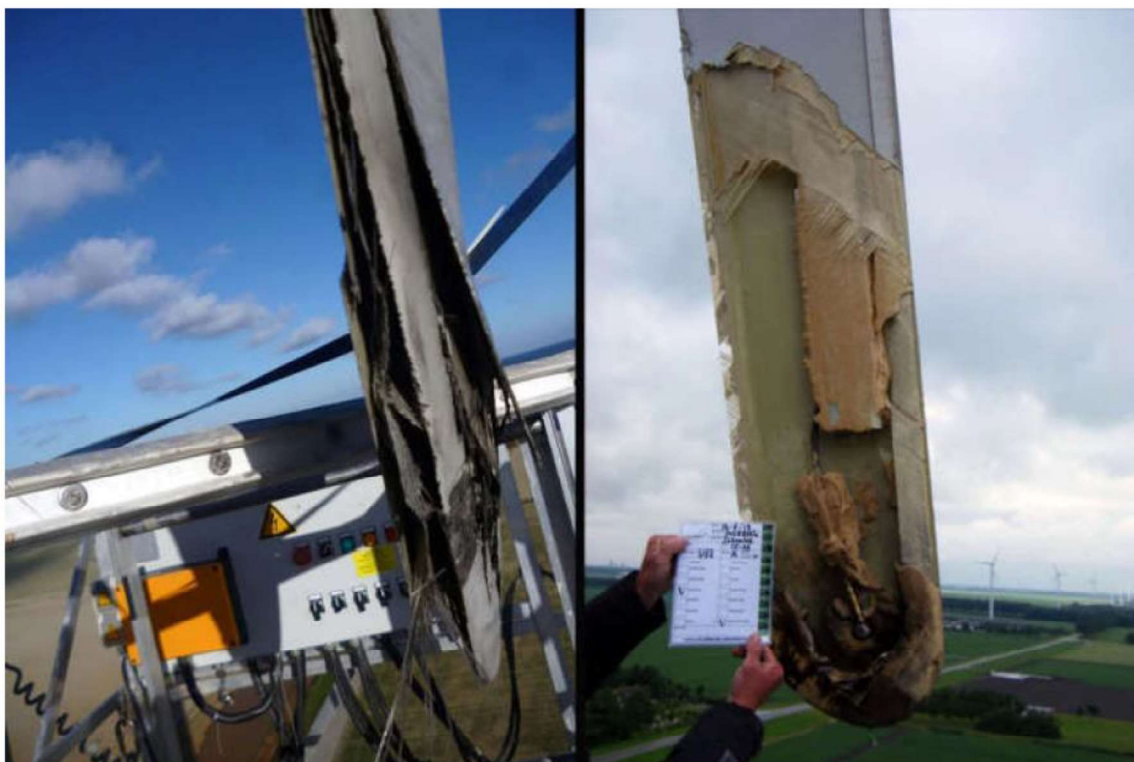
Figure 6. Images of wind turbine blade shell detachment.
