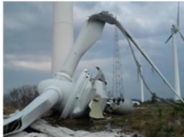
(a) Collapsed nacelle
