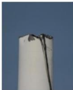
(b) Fracture section
