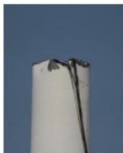
(b) Fracture section
