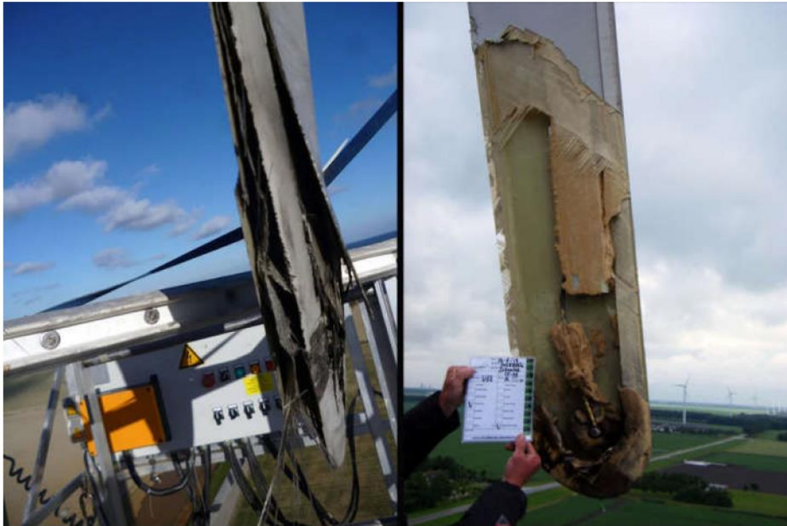
Figure 6. Images of wind turbine blade shell detachment.
