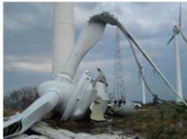
(a) Collapsed nacelle
