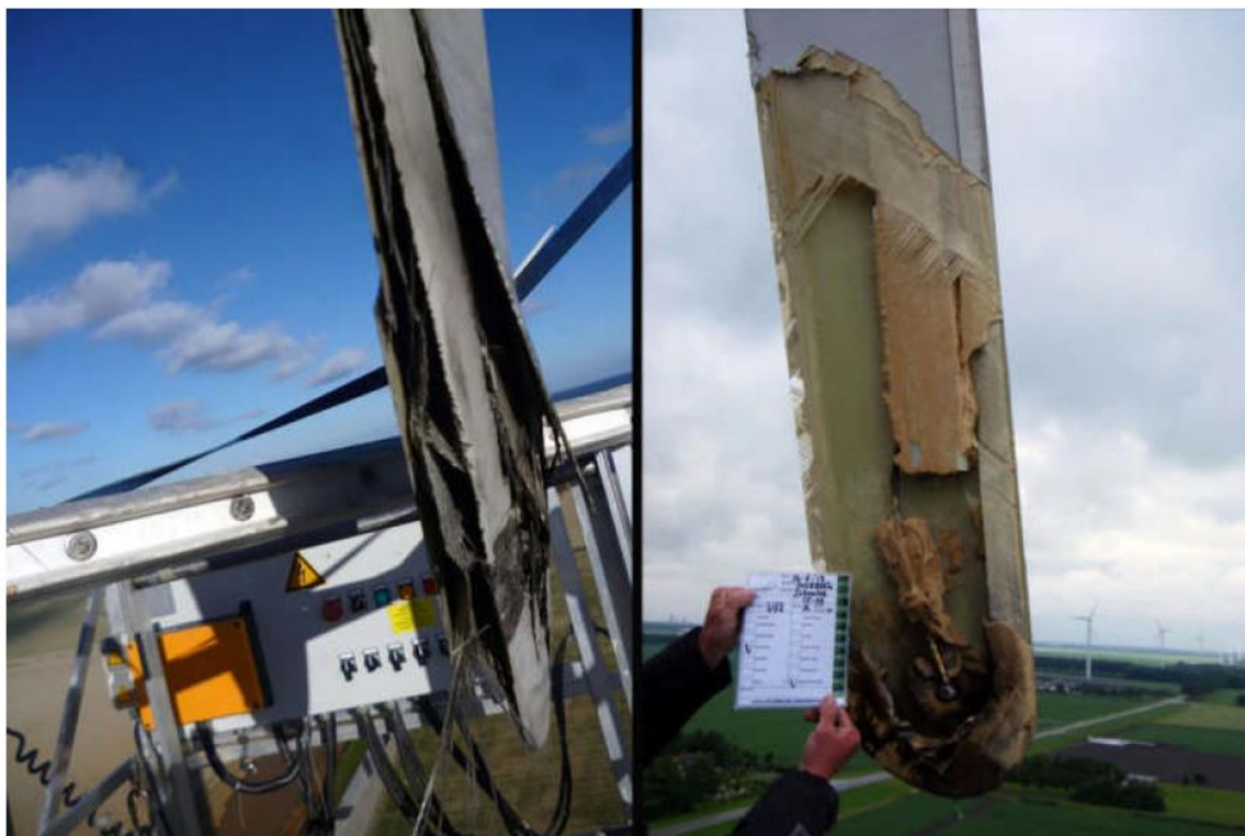
Figure 6. Images of wind turbine blade shell detachment.
