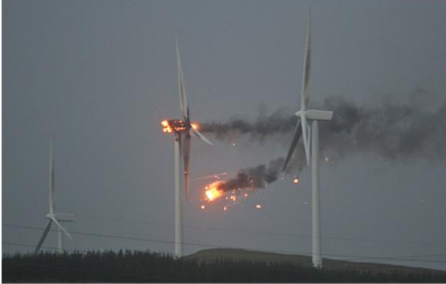
Fig. 5. Wind turbine fire at Ardrossan wind farm [17].
