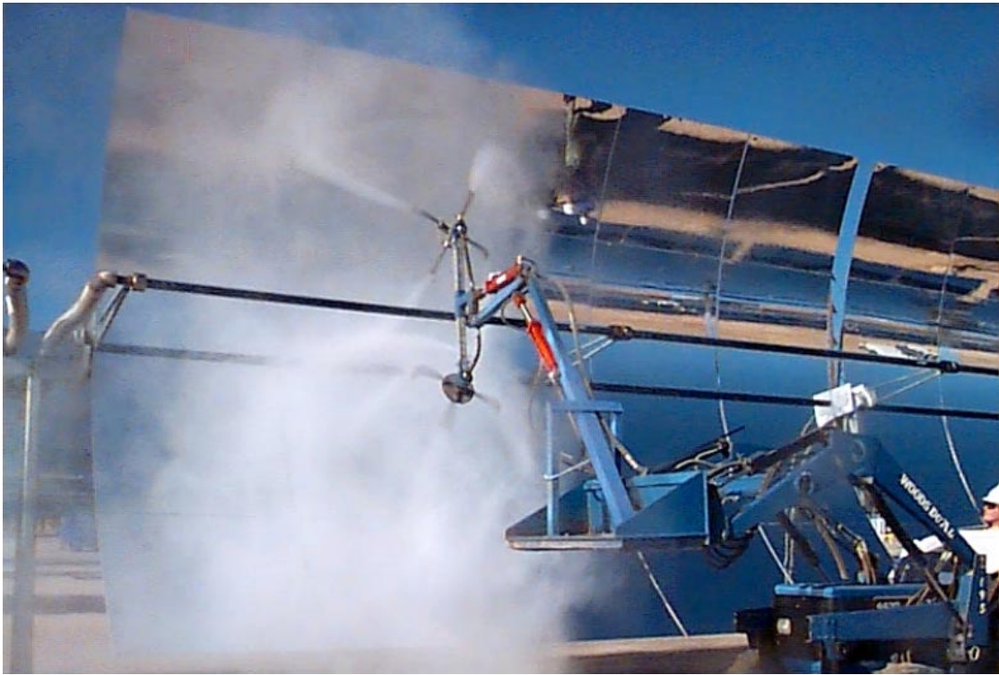
Figure 8. High-pressure demineralized water can also be sprayed on the mirrors with a new “rotating-head” rig (a.k.a. Twister) developed by the O&MIP.
