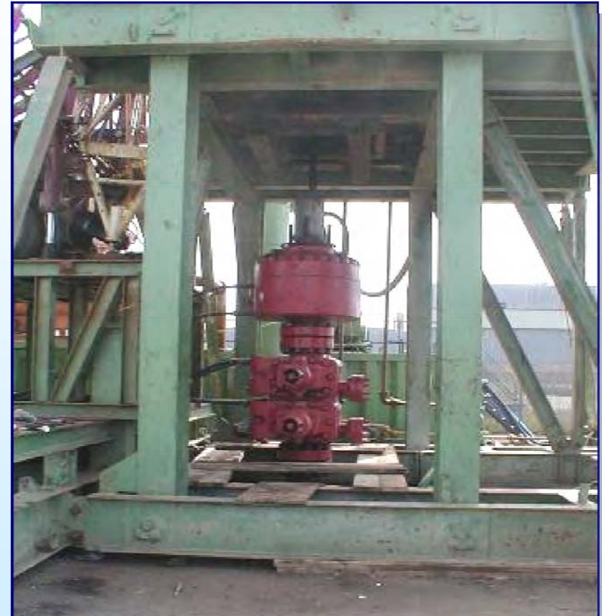
Substructure and B.O.P. stack 11" x 5000 psi
