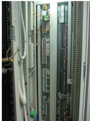
Cabinet in Substation Building
