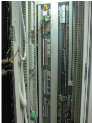
Cabinet in Substation Building
