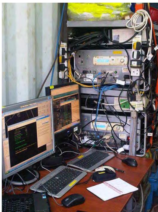
Containerised Navigation Jack Racks
