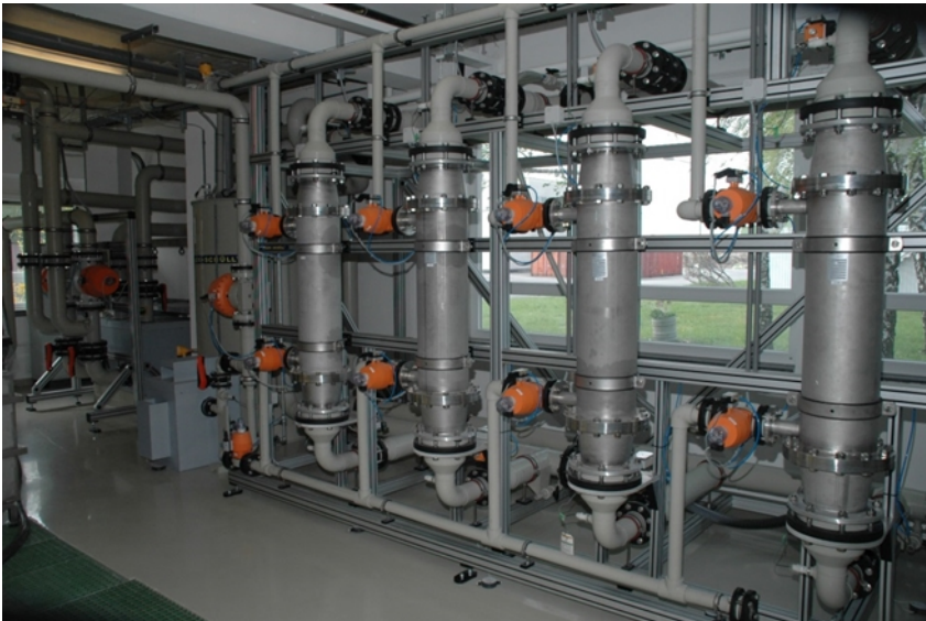
Figure 6: Filtration unit of the ultrafiltration system
