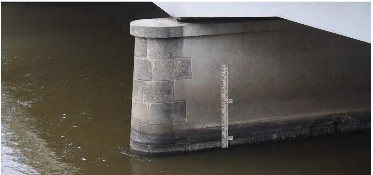
Staff gauges installed on bridge pillar
