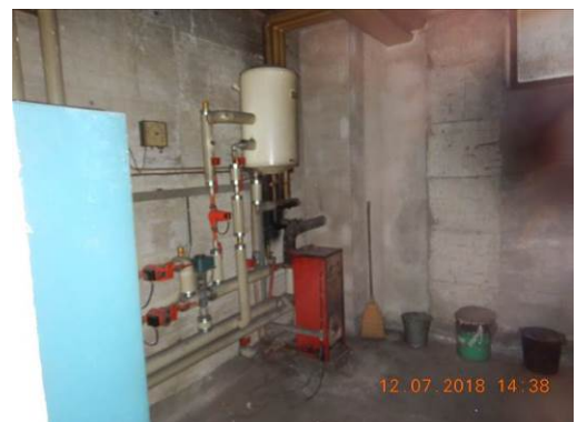
Locale caldaia – Piano interrato
