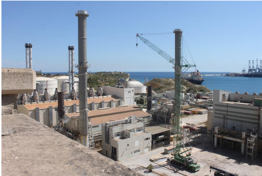
Figure 9: Enemalta power station
