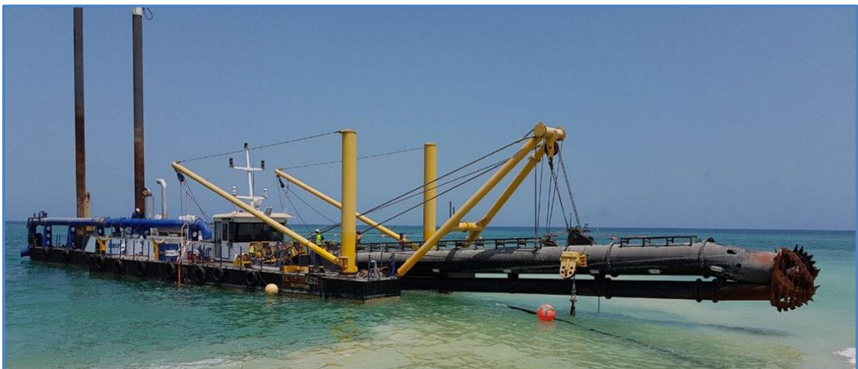
Figure 4.2 – Preparation Works at HDD Offshore Bore Hole Exit – Example of Cutter Suction Dredger Vessel
