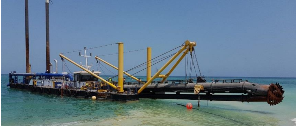
Figure 12: Preparation Works at HDD Offshore Bore Hole Exit – Example of Cutter Suction Dredger Vessel
