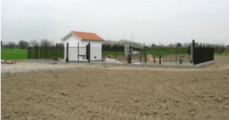
Figure 10: Example of Block Valve Station
