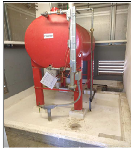
Serbatoio motopompa 1 m 3
