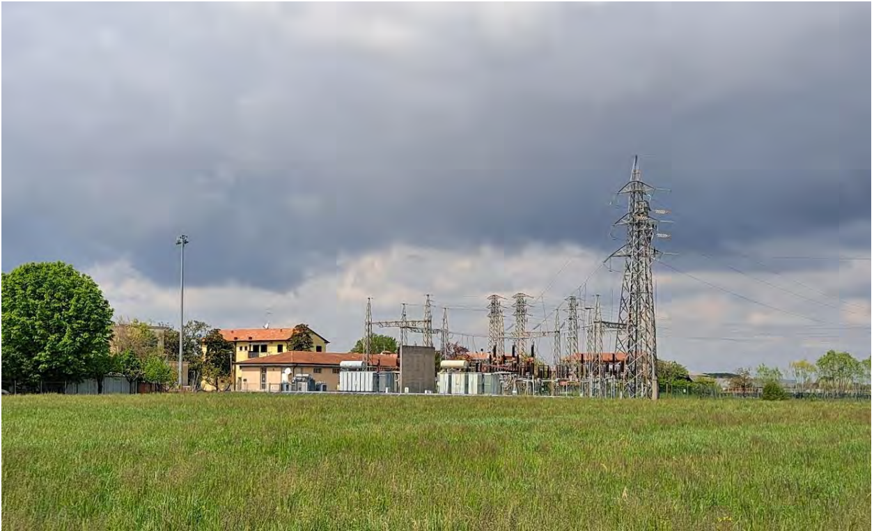
Figura 5-31 – Cabina primaria AT/MT “Levada”
