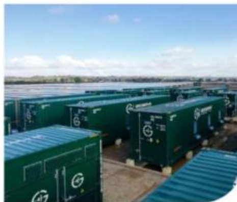
27.5MW/30.14MWh PV+ESS Yorkshire, England 🇬🇧
