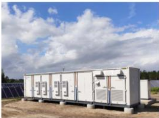
1.5MW / 3.836MWh DC-coupled Energy Storage Project in Florida, USA 🇺🇸
