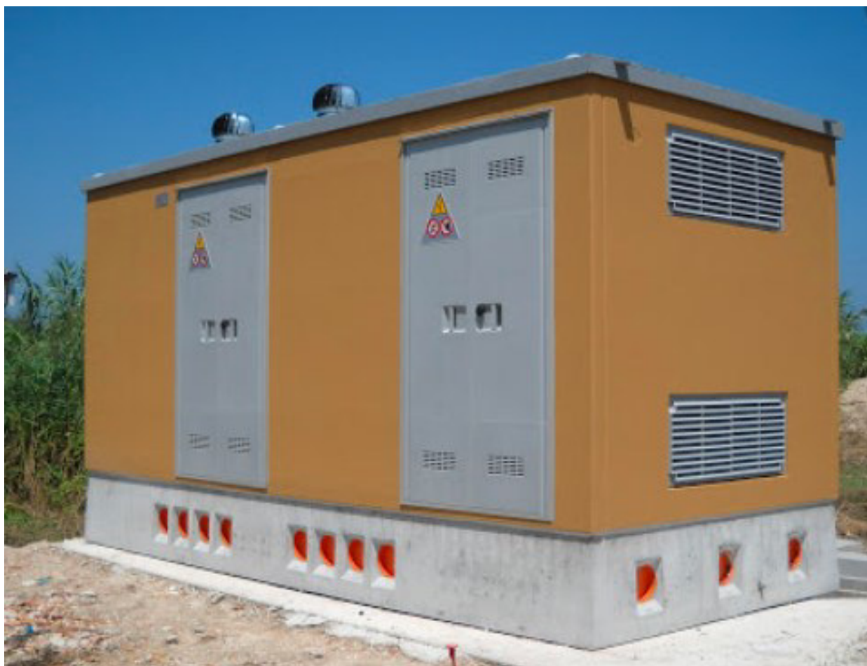
Figura 11 - Cabine in CAV
