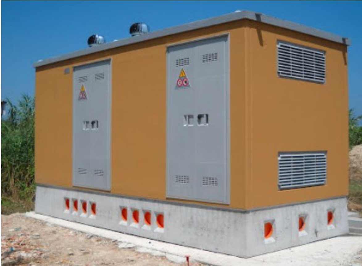
Figura 4 - Cabine in CAV
