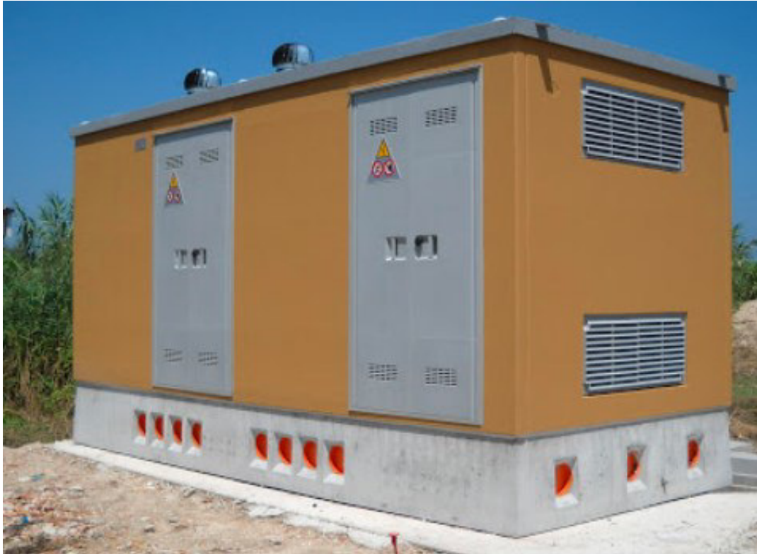
Figura 8 - Cabine in CAV
