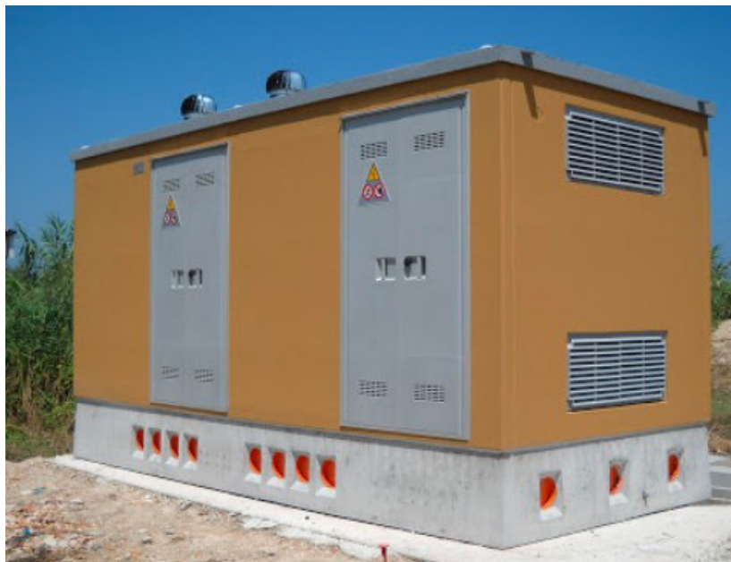
Figura 6 - Cabine in CAV
