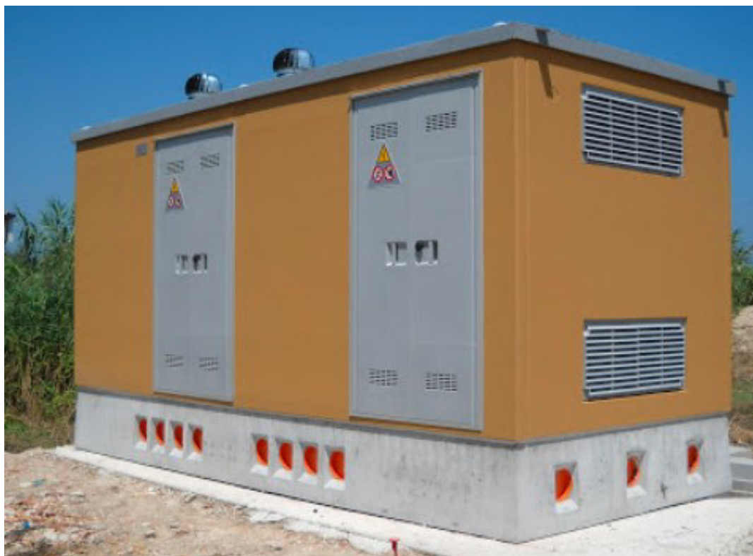
Figura 2 - Cabine in CAV
