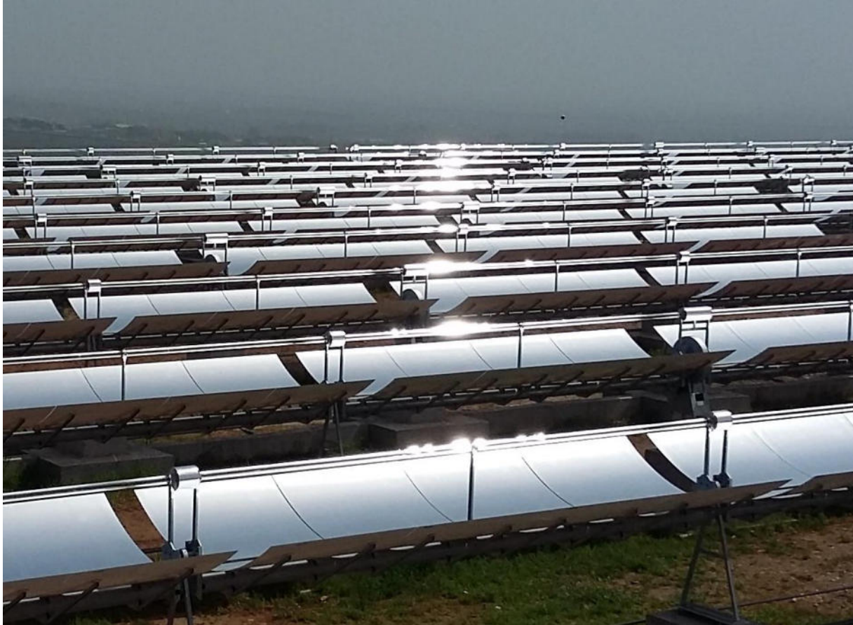
Tunisia – PTMx - Power generation
