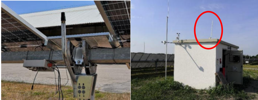
TP's antenna on the tracker (left) and RP's main antenna on the top of the transformer station (right)
