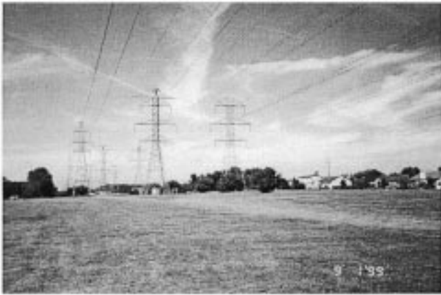
Fig. 2. Multiple line easement with double circuit 120-kV, 345-kV, and 345-kV transmission lines.
