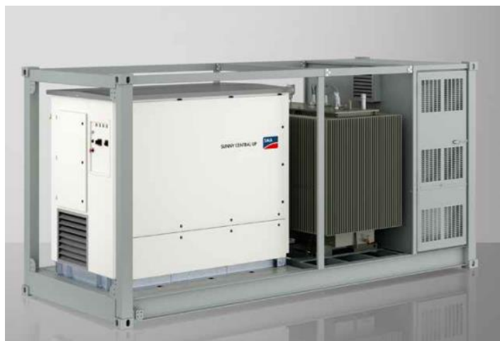
Fig.8: MV POWER STATION
