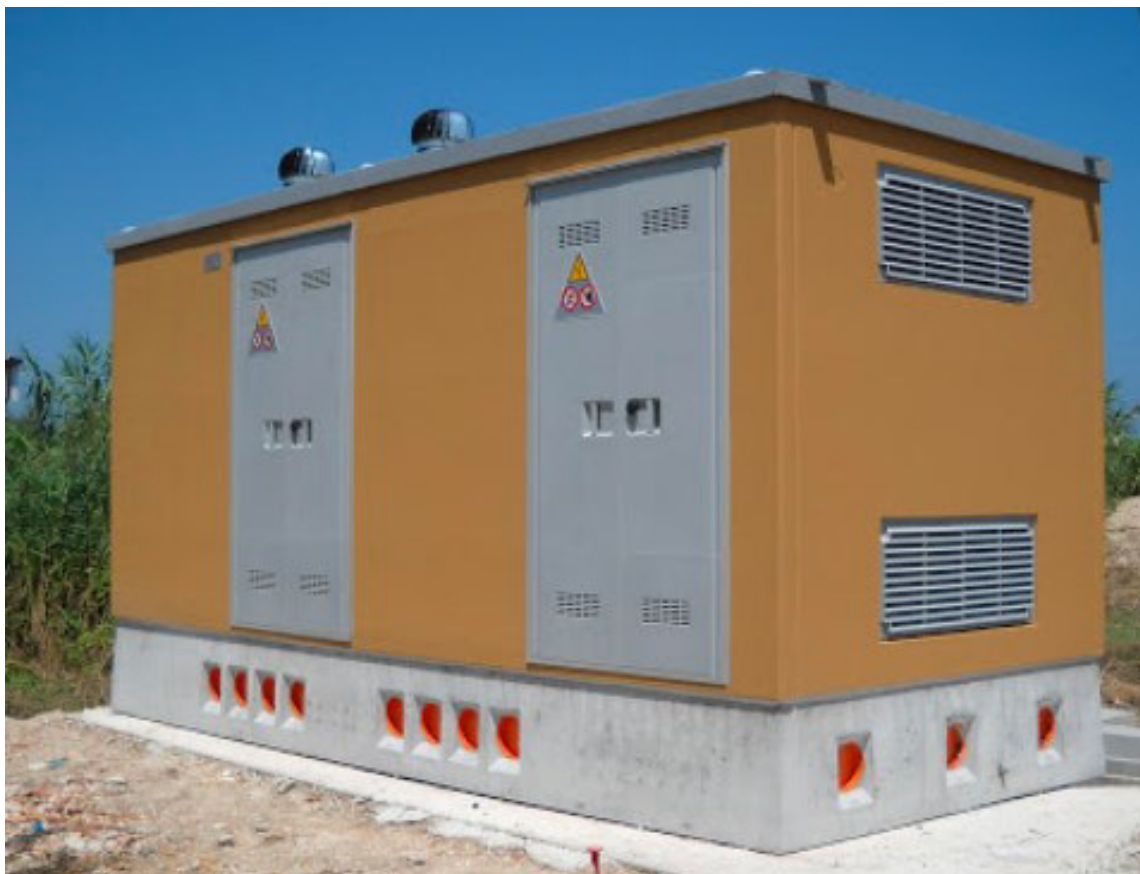
Figura 6 Cabine in CAV
