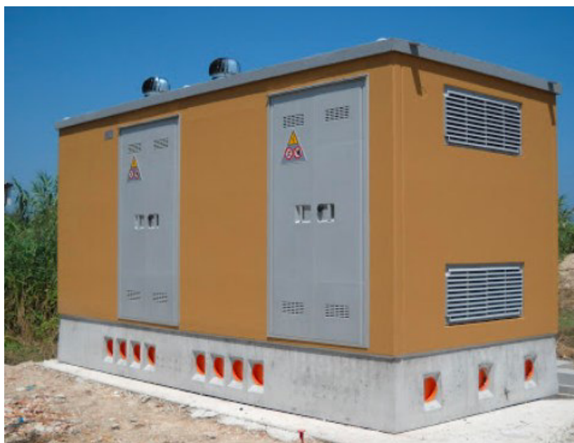
Figura 6 - Cabine in CAV
