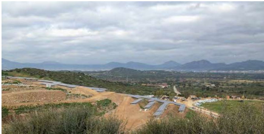
Fig. 14. 1 MW p photovoltaic system at landfill Spiritu Santo. In order to create suitable condition for reconstituting a damaged ecosystem, the system has been designed with the consultancy of landscape designers by CIPNES (an administrative body devoted to the planning of industrial areas). Image courtesy of CIPNES.
