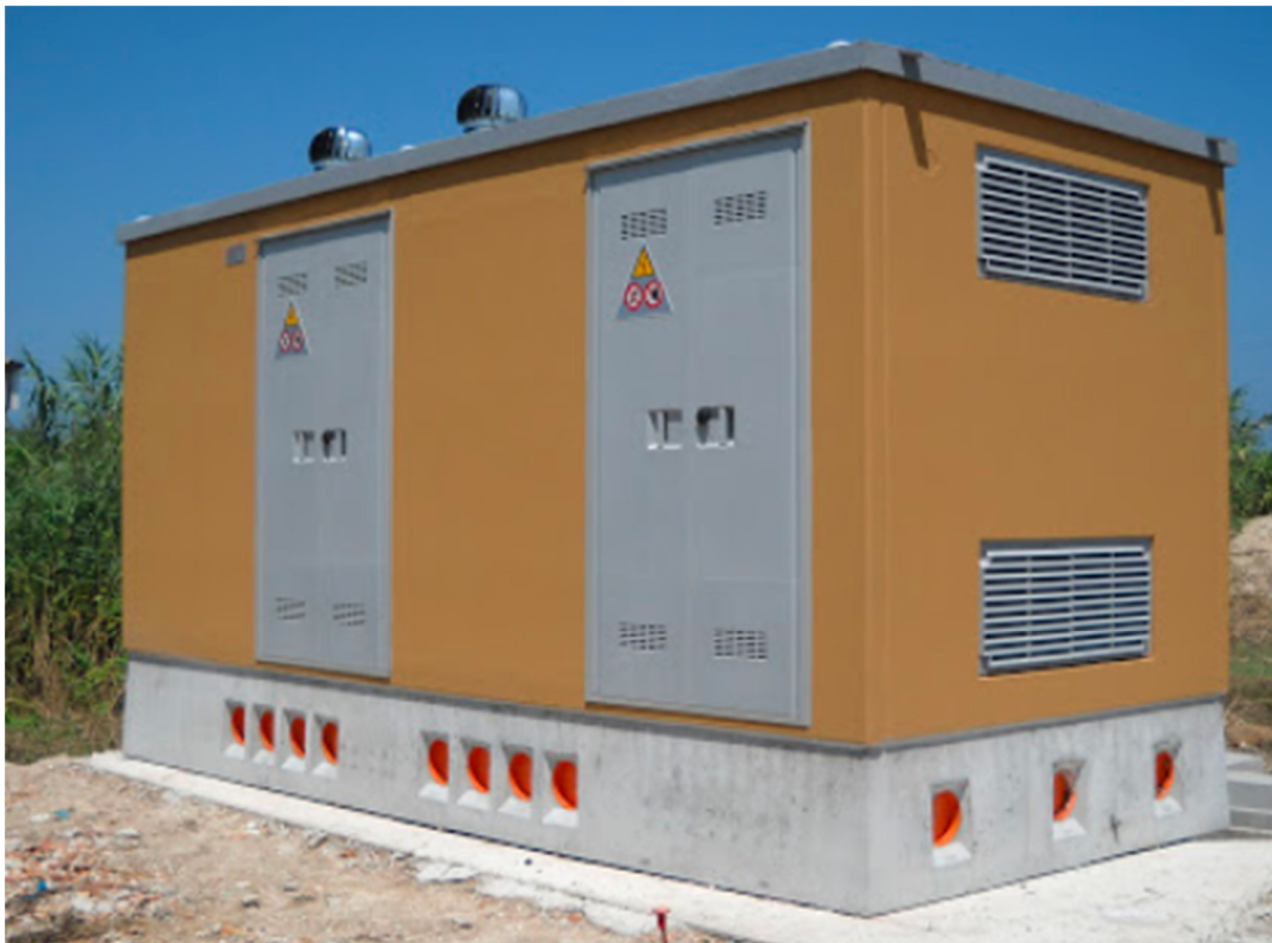
Figura 5 - Cabine in CAV
