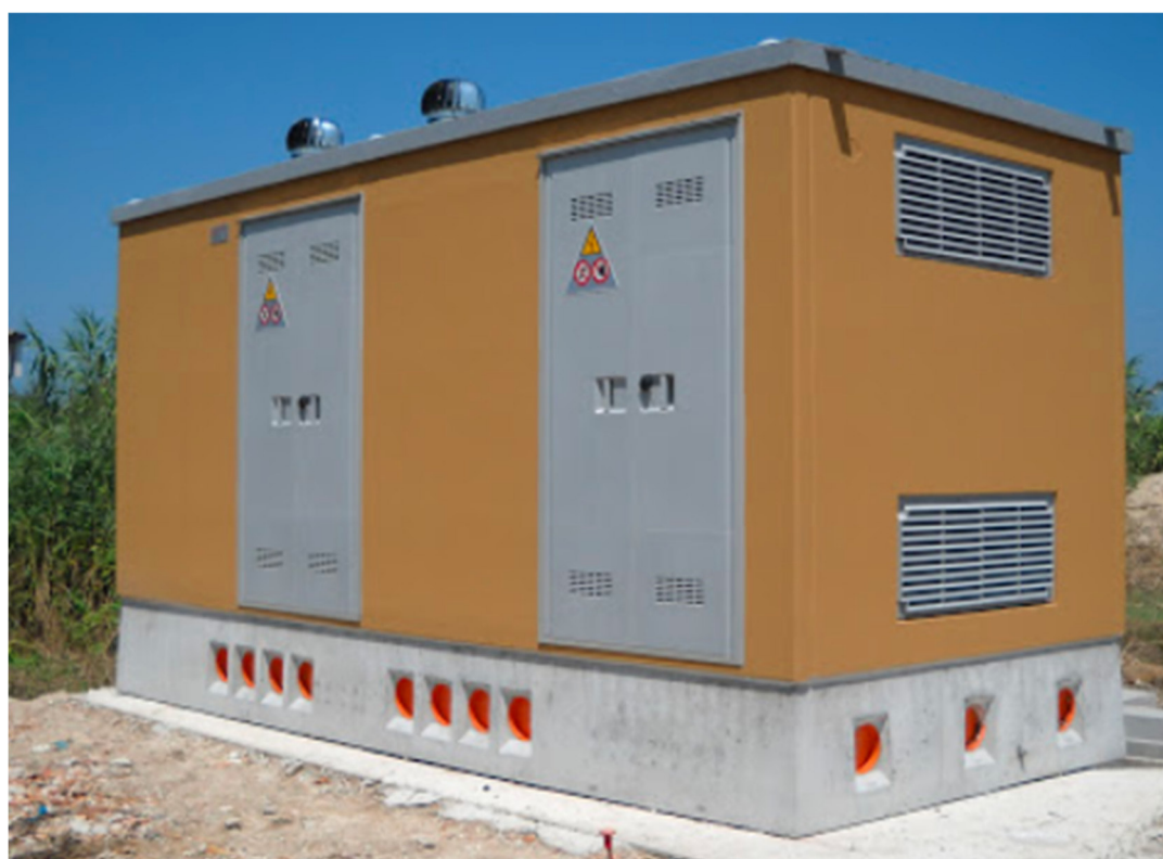
Figura 7 - Cabine in CAV
