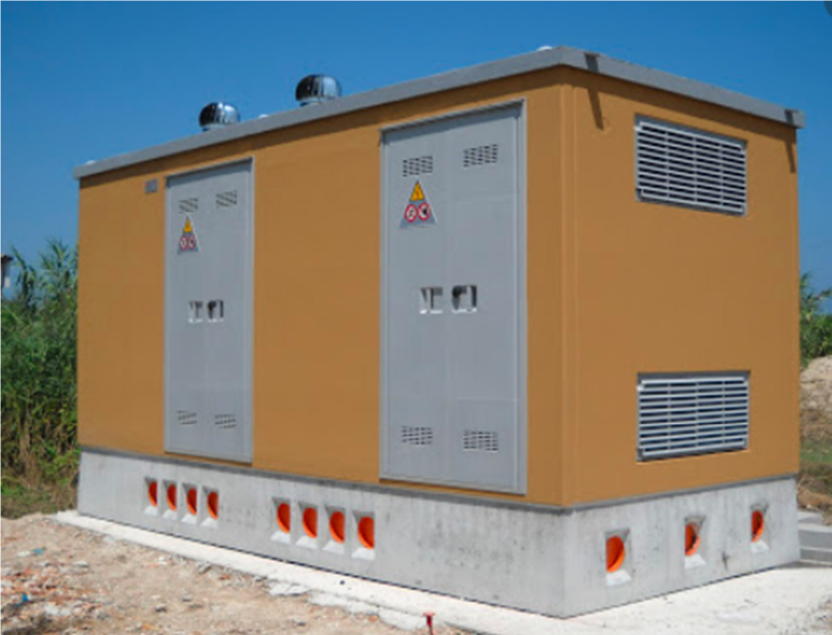
Figura 16 - Cabine in CAV
