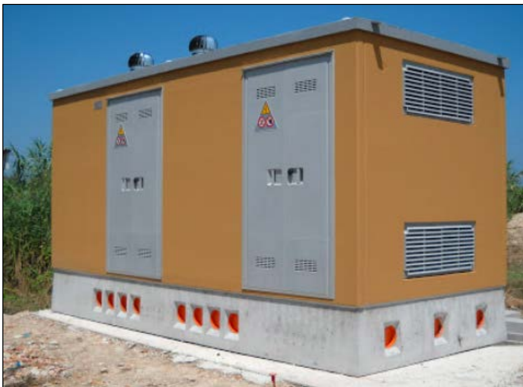
Figura 13 cabina in CAV
