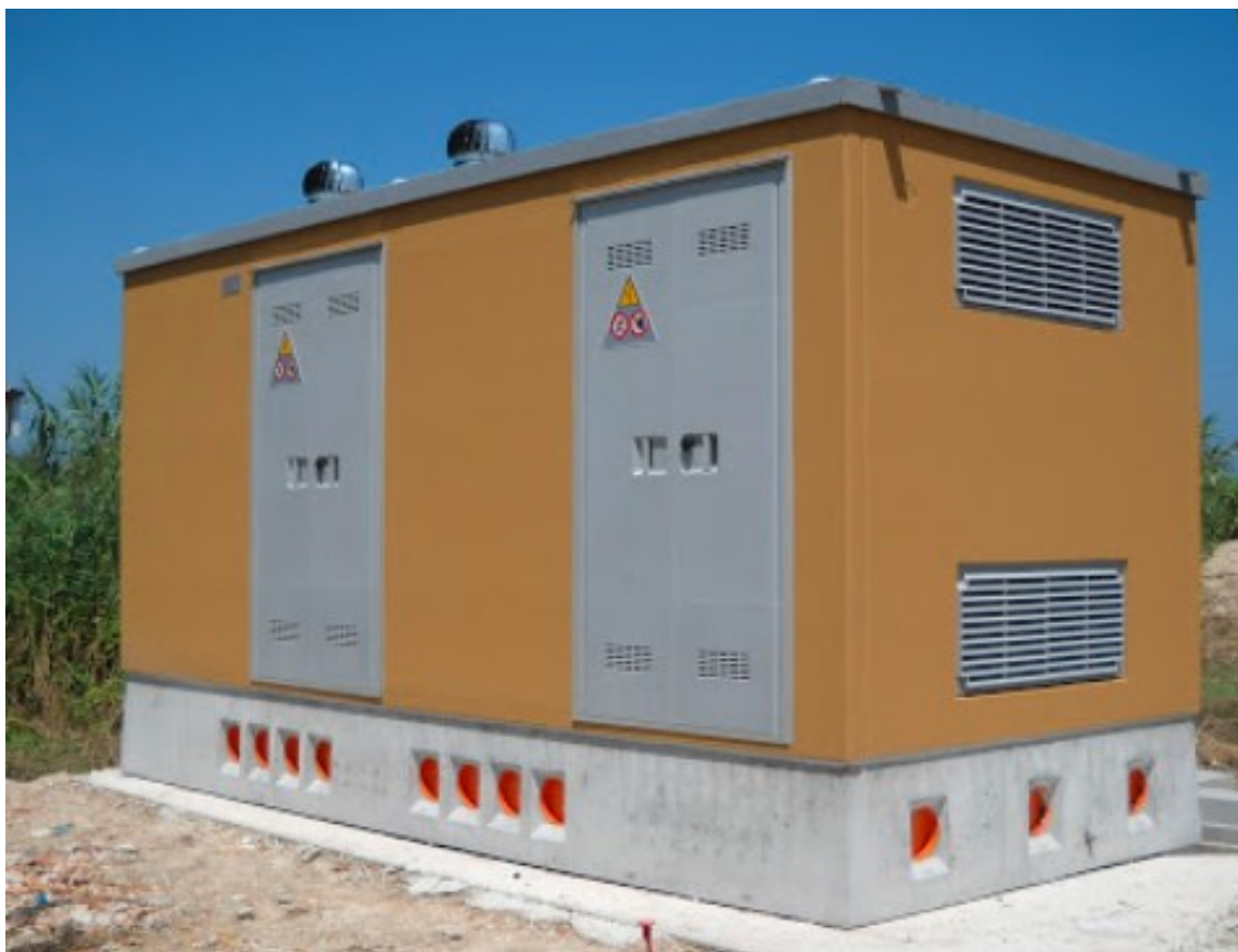
Figura 3 Cabine in CAV
