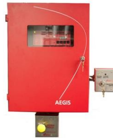
Fire suppression control panel
