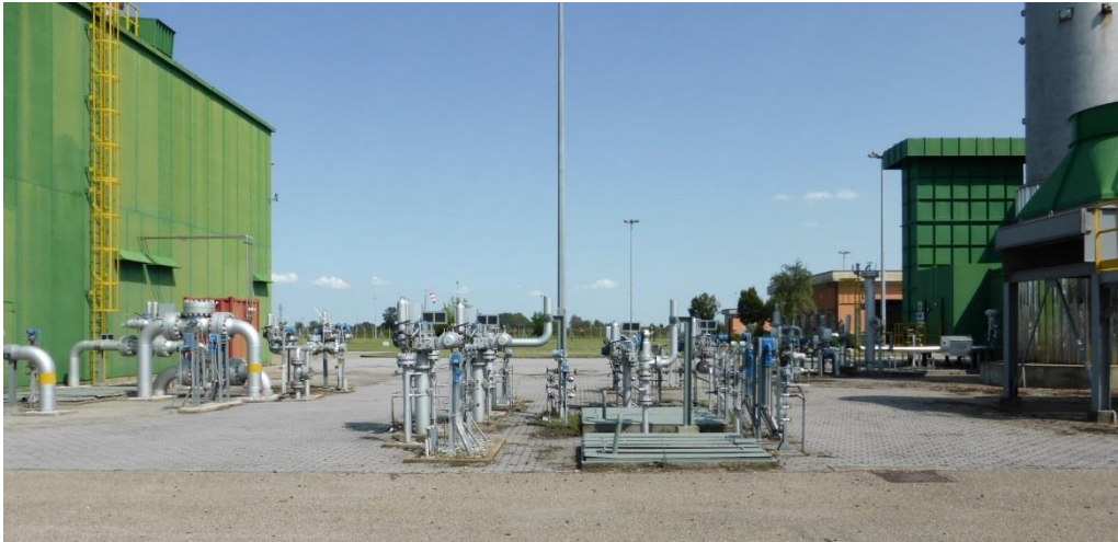
Figure 17: Pipework Between Compressor Enclosures
