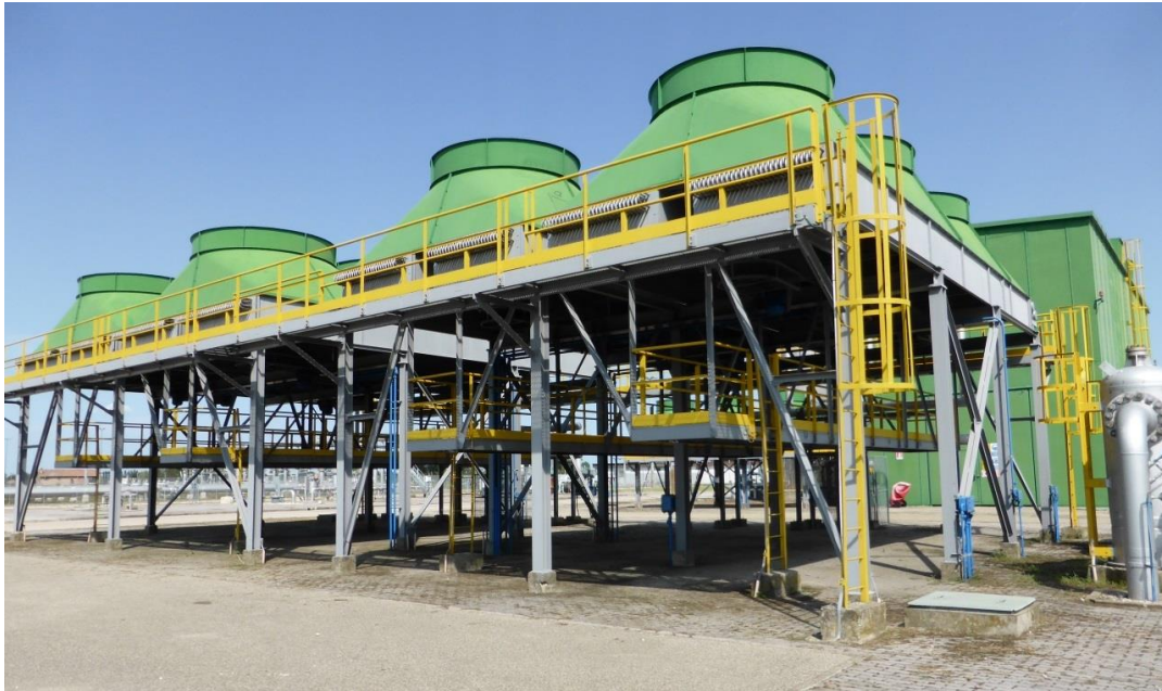
Figure 18: Air Cooler in Compressor Area
