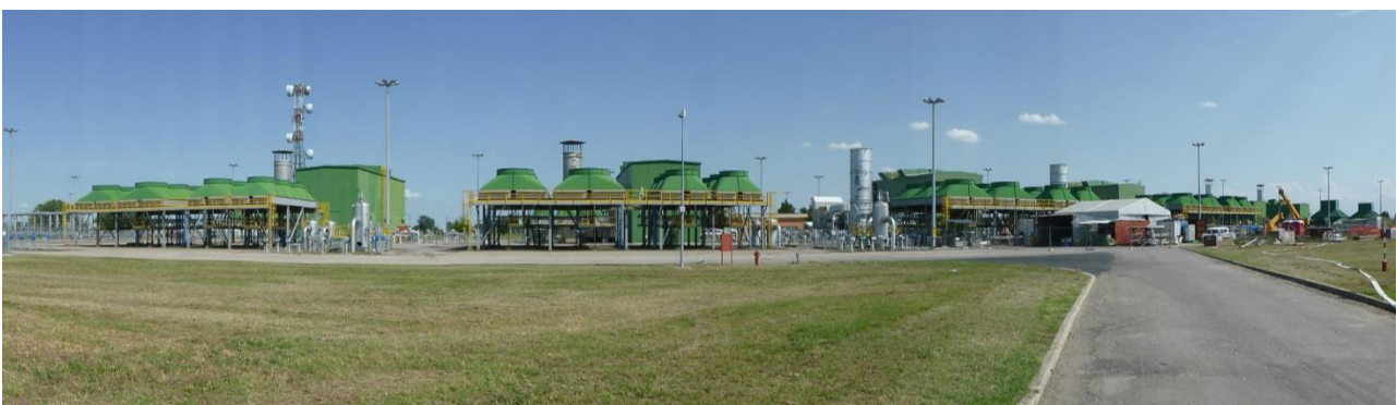
Figure 16: Compressor Area of the Minerbio Site
