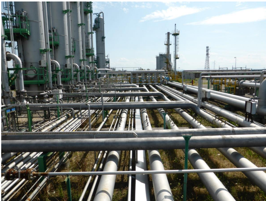
Figure 20: Pipework Adjacent to Dehydration Towers
