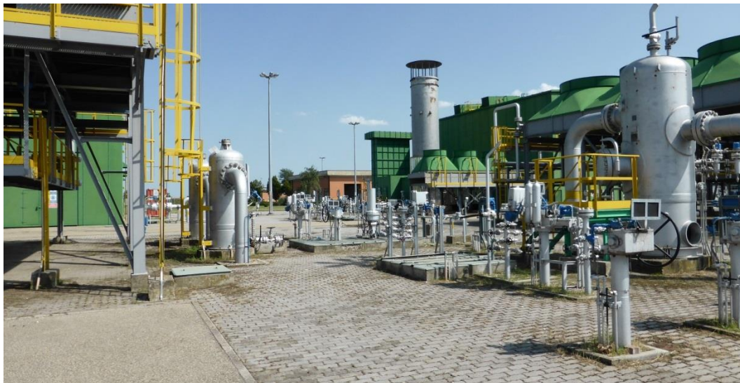
Figure 19: Pipework Adjacent to the Air Coolers
