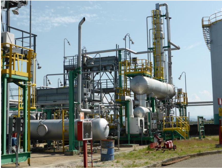
Figure 21: Process Unit in Dehydration Area
