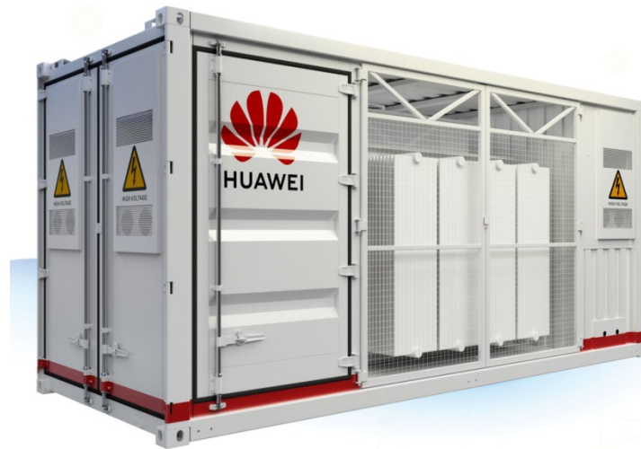
Figura 5 – Smart Transformer Station
