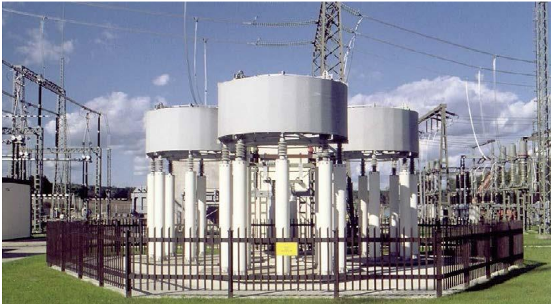
Figura 35 - shunt capacity reactor - fonte Siemens
