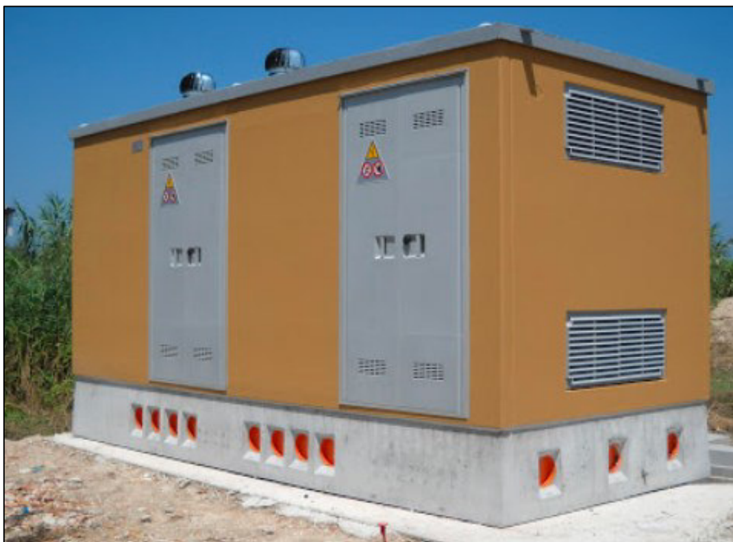
Figura 19 cabina in CAV
