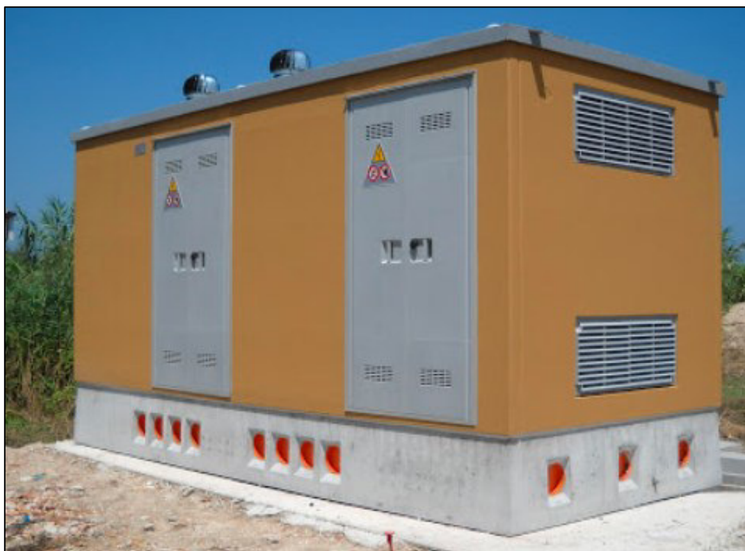
Figura 5 cabina in CAV
