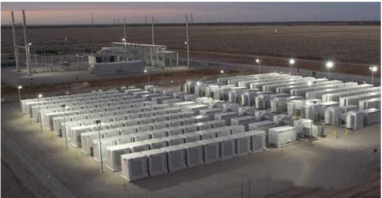
Storage Enel Greenpower
