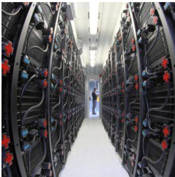
Fig. 3.30 – Storage (BESS) interno del container
