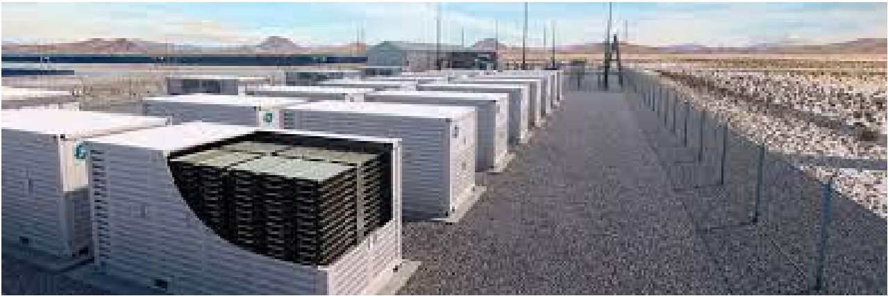
Fig.3.29 – Storage (BESS) in container in aree dedicate
