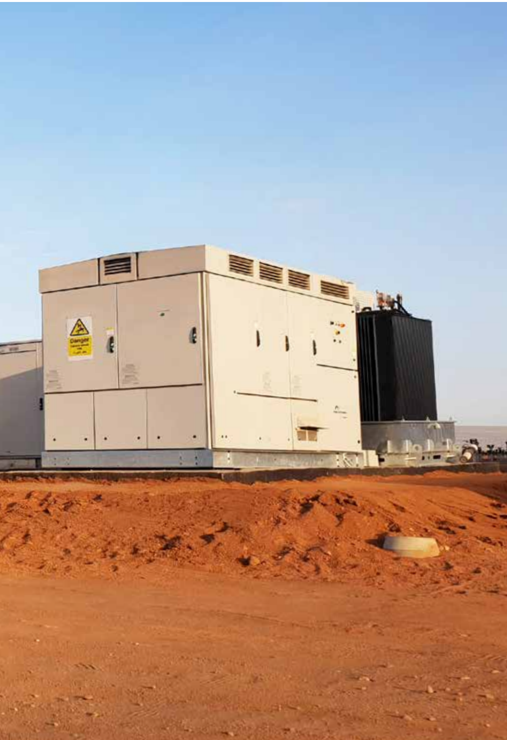
HEMK + TWIN SKID Egypt - Alcazar PV plant (283MW)
