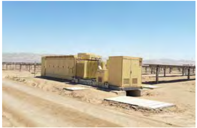
CHILE Uribe, 50 MW HEC PLUS + MV SKID
