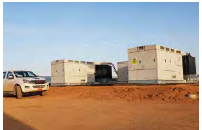
EGYPT Alcazar, 283 MW HEMK+ TWIN SKID
