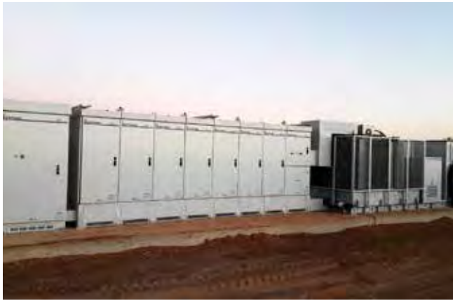
JORDAN Al Mafrq, 61 MW HEC V1500 + MV SKID JORDAN'S 1 ST 1500V INVERTER
