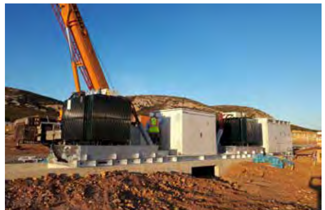
SPAIN La Nava, 46 MW HEMK + TWIN SKID
