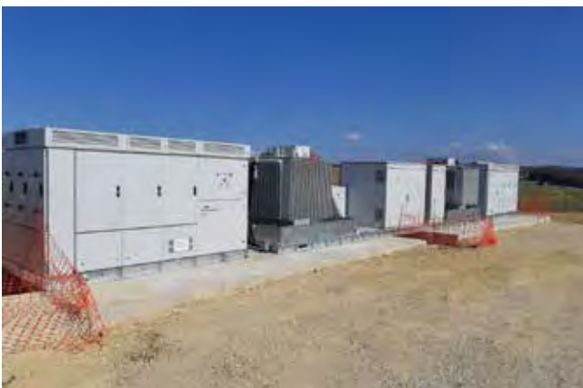
SPAIN Guillena, 105 MW HEMK+ TWIN SKID
